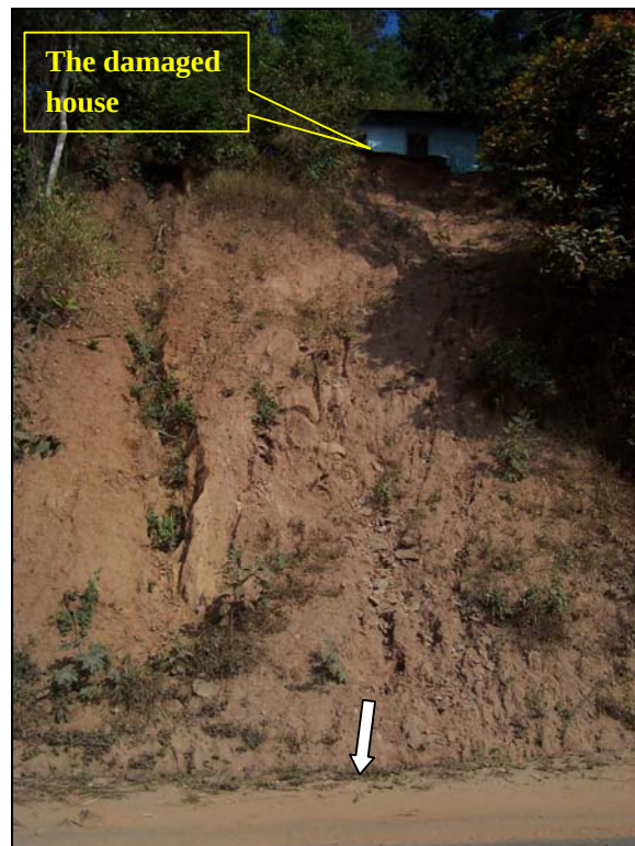
Photo 5: The damaged house standing in the mid slope of the slide, rills formed all over the slide zone.
