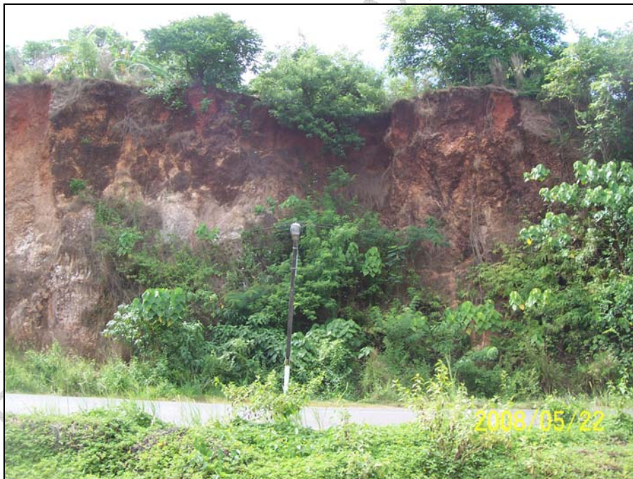
Photo 120: The plan view of the debris slump with steep slope angle
