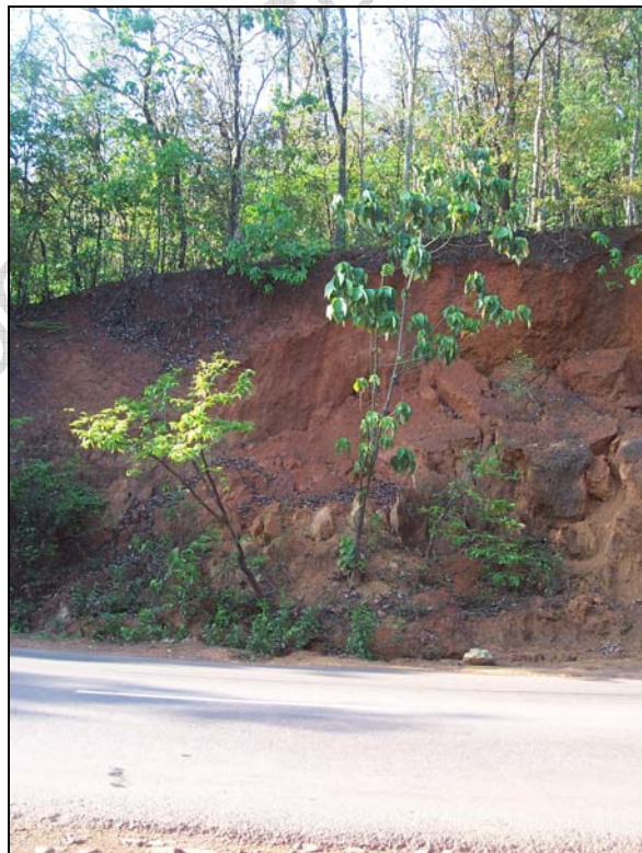
Photo 111: The side view of the debris slide with slided material at the toe.
