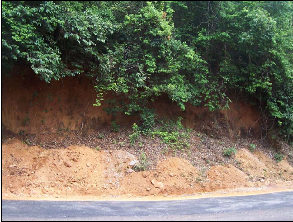
Photo 80: The view of the debris slump with unstable crown.
