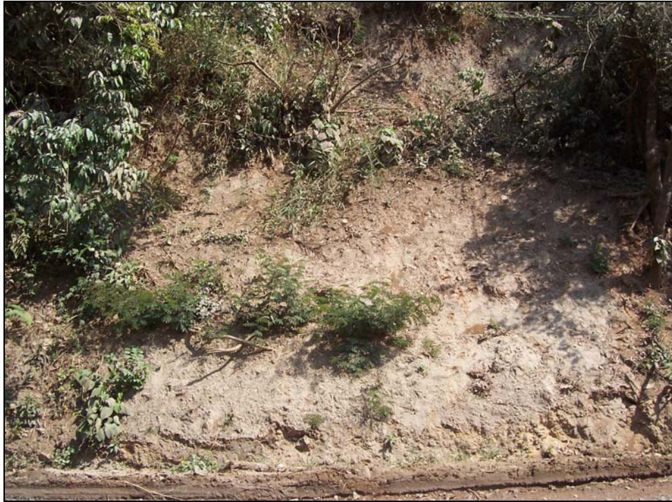
Photo 23: The plan view of the debris slide with exposed bed rock.
