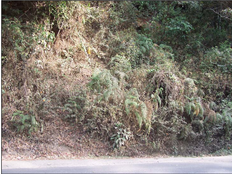
Photo 51: The old debris slump covered by small trees
