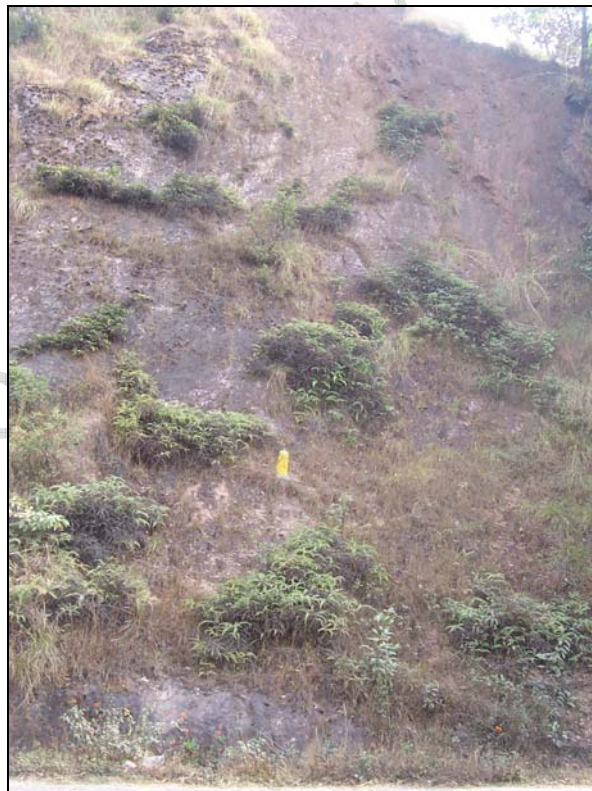
Photo 50: View of the debris slump exposing the bed rock over which it has moved.
