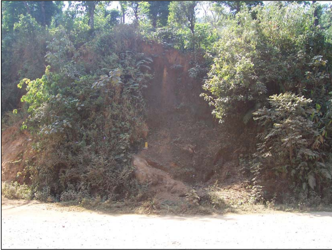
Photo 27: The plan view of the debris slide with unstable crown.
