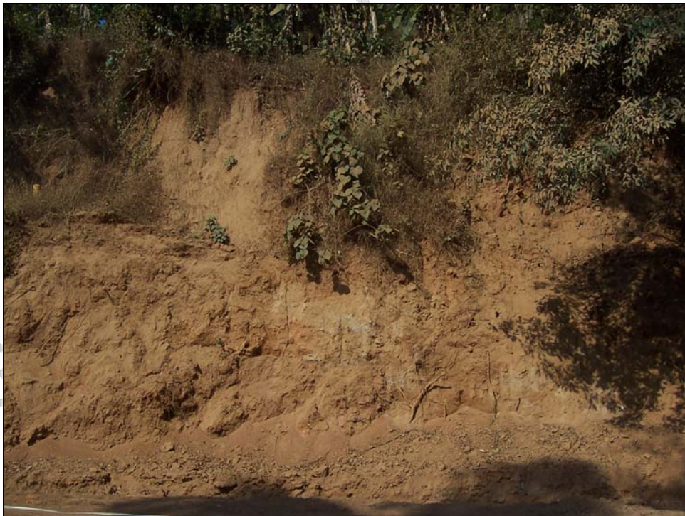
Photo 35: The plan view of the debris slide with unstable crown
