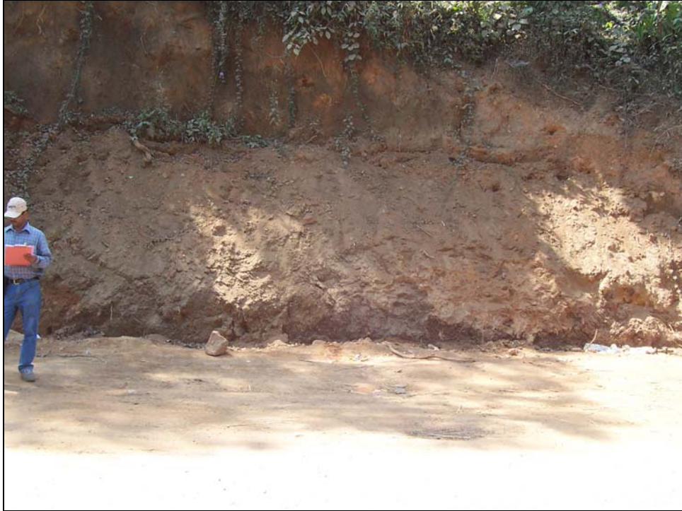
Photo 28: The plan view of the debris slide with unstable crown.
