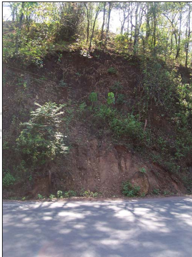
Photo 99: The view of the debris slide with unstable crown
