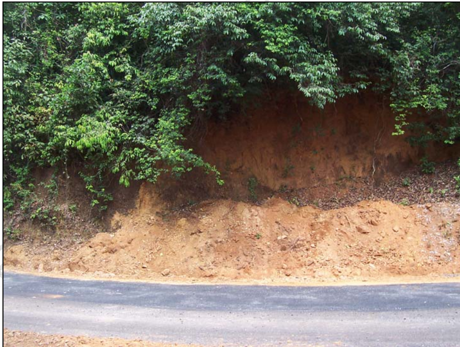
Photo 81: The view of the debris slump with unstable crown.
