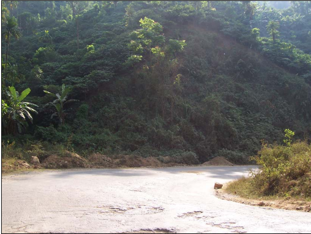
Photo 40: The plan view of the debris slide covered by plants
