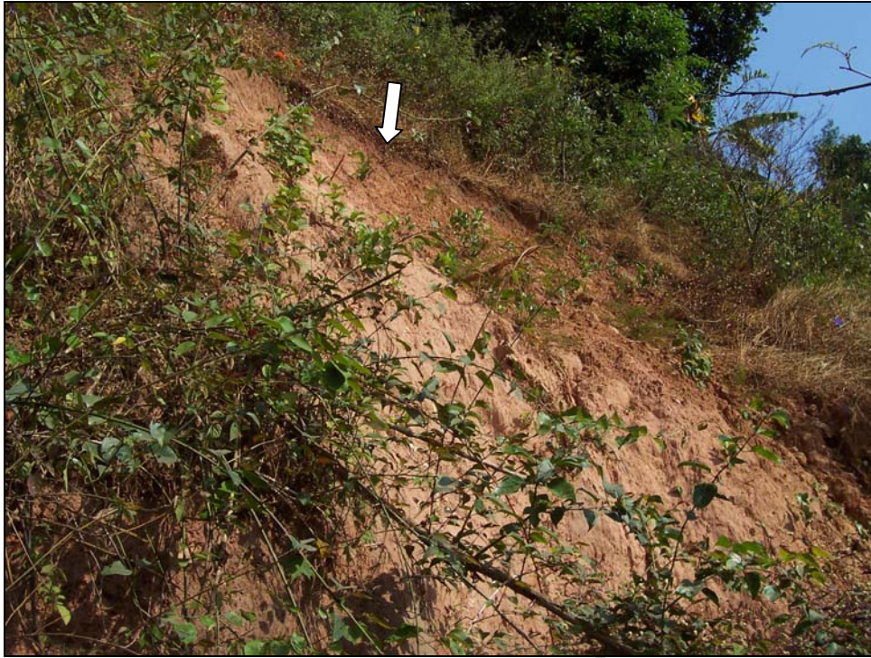
Photo 7: The land slide in the vertical cut slope with scar at the back of the house
