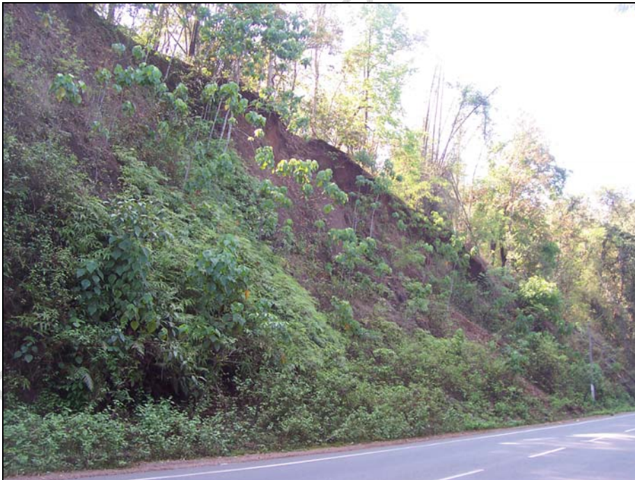
Photo 103: The side view of the reactivated debris slide.
