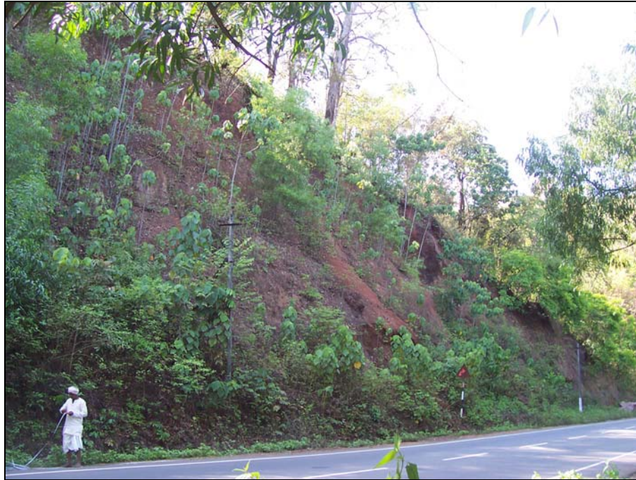
Photo 100: The side view of the debris slide with unstable crown
