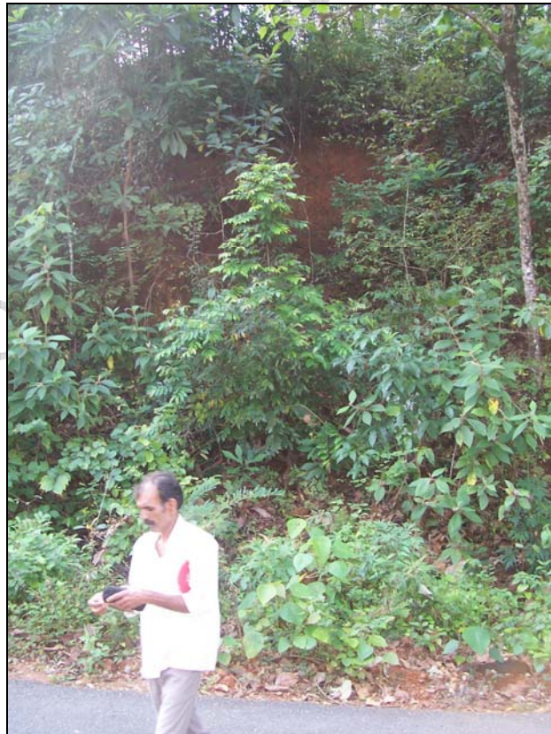
Photo 67: The plan view of the debris slide with exposed bed rock
