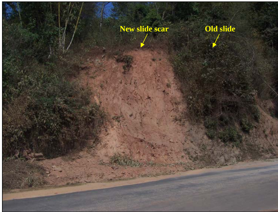
Photo 13: Lateral progradation of the slide along SH88 cut slopes
