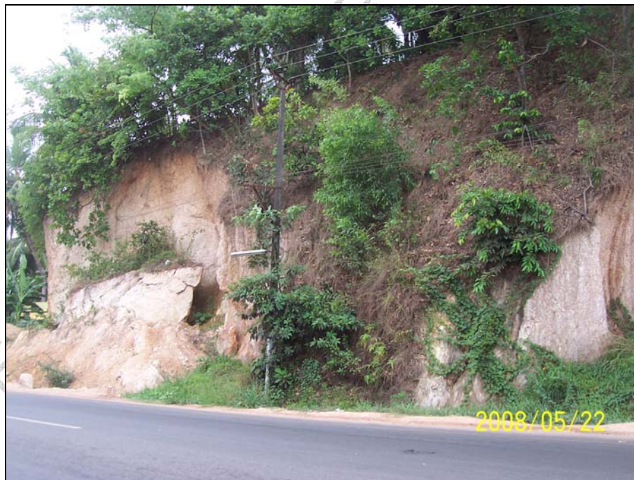
Photo 122: The side view of the debris slump with steep slope angle
