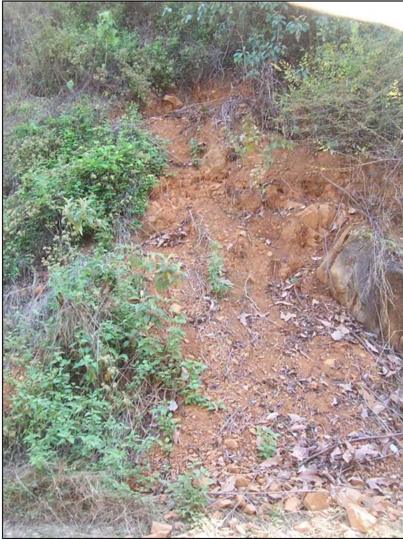
Photo 73: The plan view of the debris slump with slided material in the slope.
