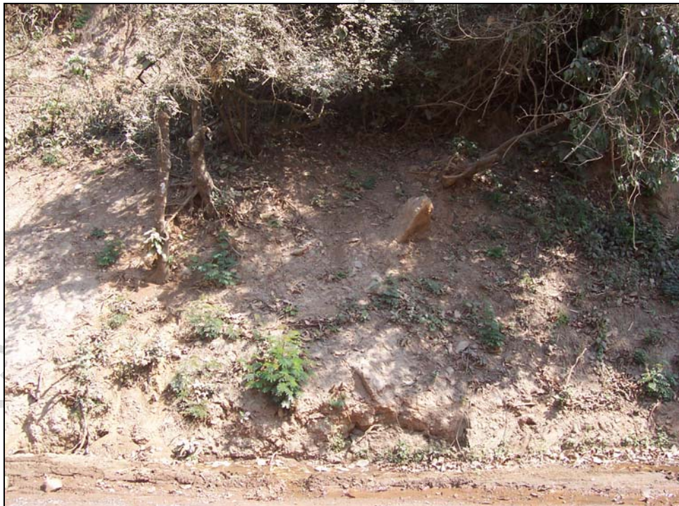
Photo 24: The plan view of the debris slide with exposed bed rock.
