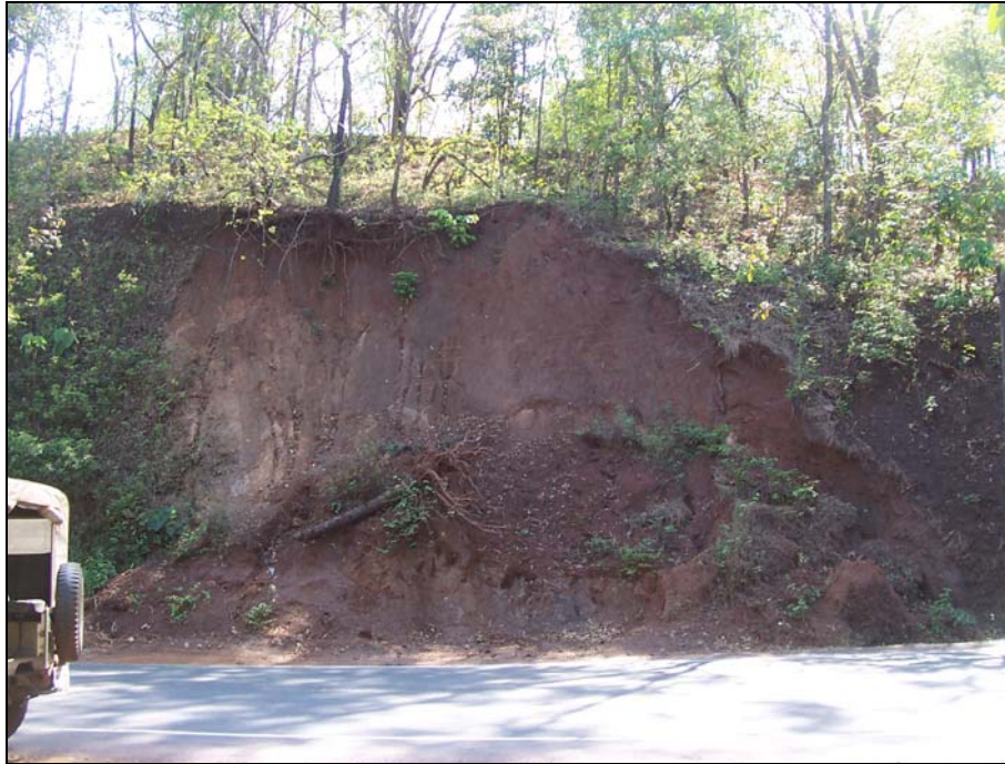
Photo 98: The view of the debris slide with unstable crown
