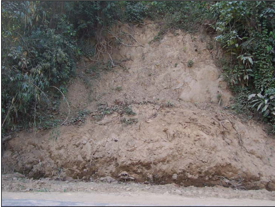
Photo 36: The plan view of the debris slide with unstable crown
