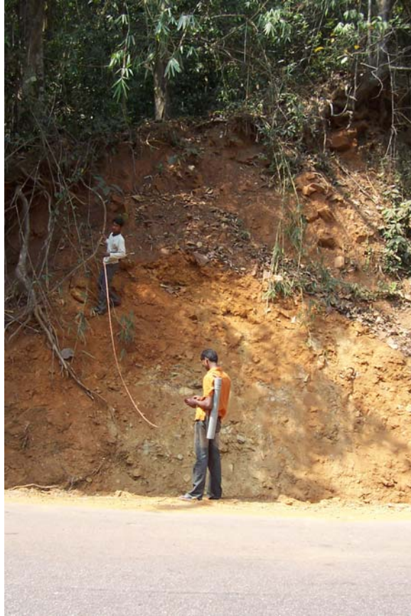
Photo-114: view of the debris slide with slided material
