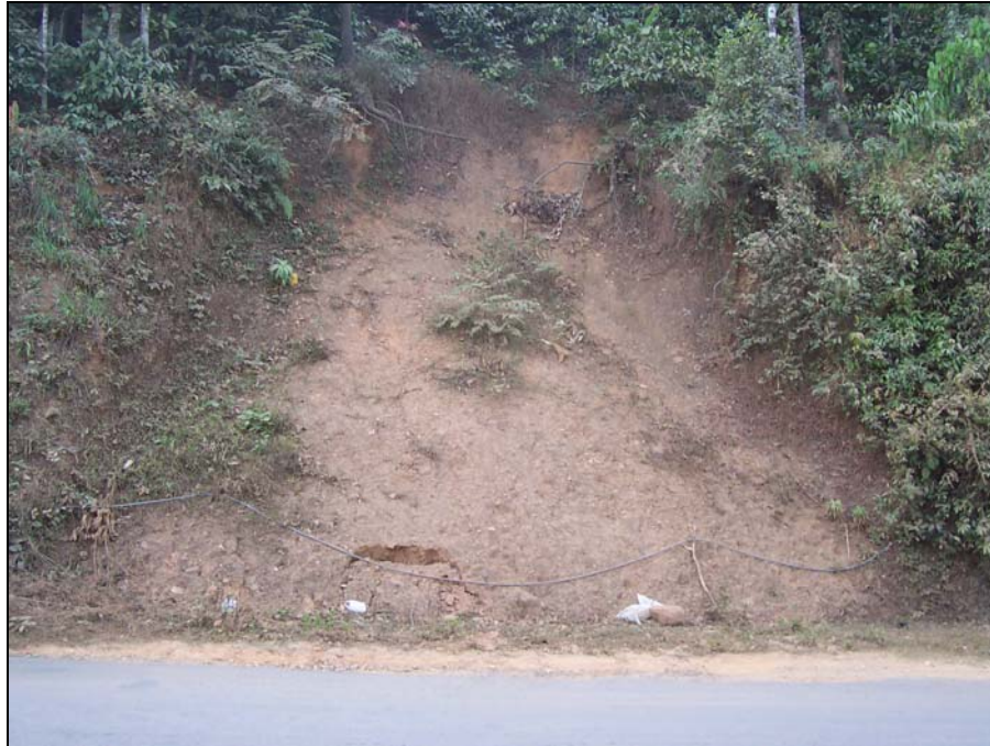
Photo 41: The plan view of the debris slide with unstable crown
