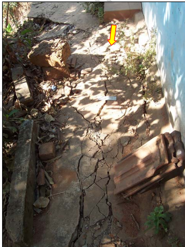
Photo 6: The arrow shows the damaged pavement with crown cracks
