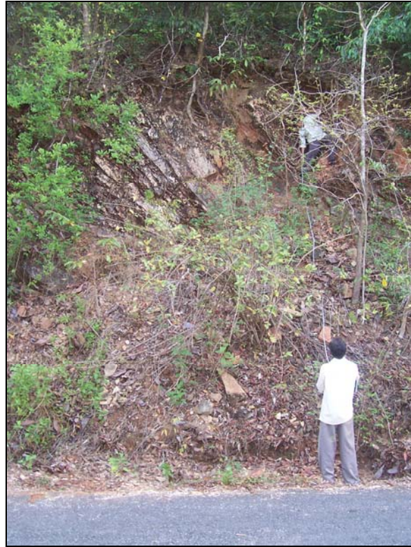
Photo 60: The plan view of the reactivated rock slide along day lighted plane.
