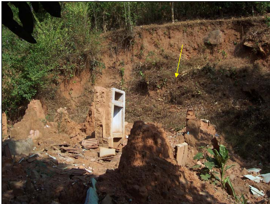
Photo 10: The damaged house which was located along the run out path of the slide
