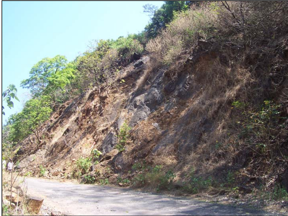
Photo 78: The view of the rock slide with unstable crown.
