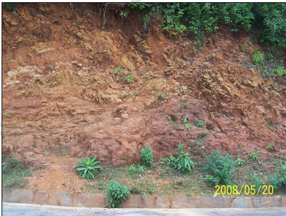
Photo 116: The plan view of the debris slump
