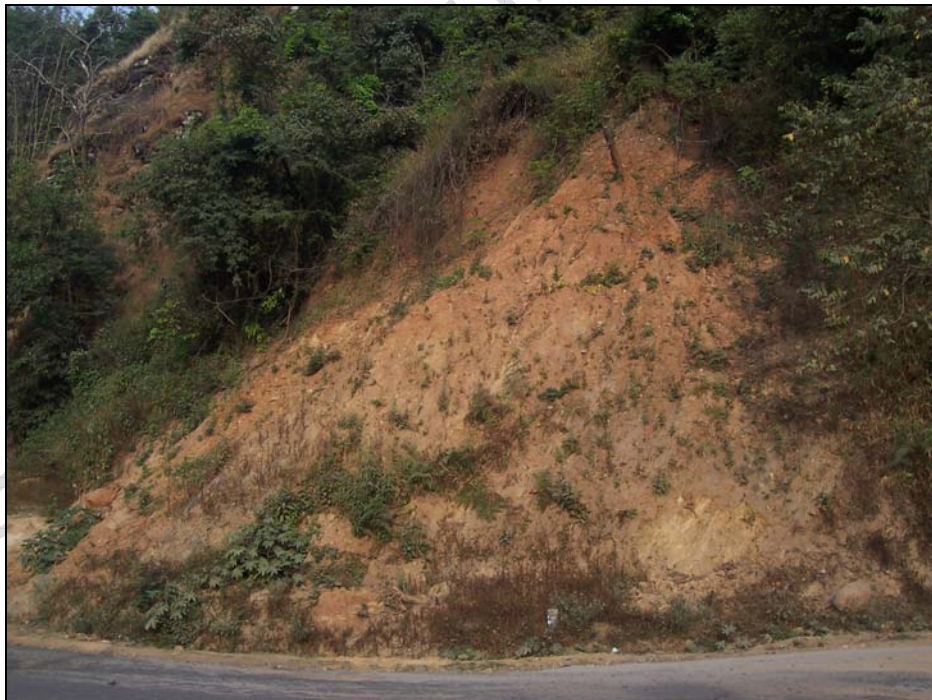
Photo 44: Side view of the reactivated slide with exposed weathered granite
