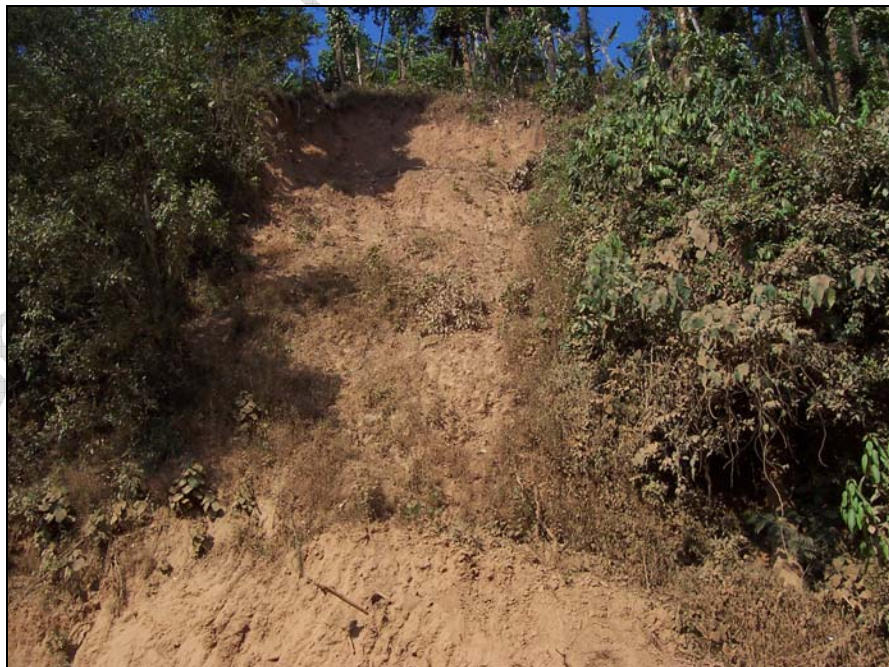
Photo 33: The plan view of the debris slide with unstable crown
