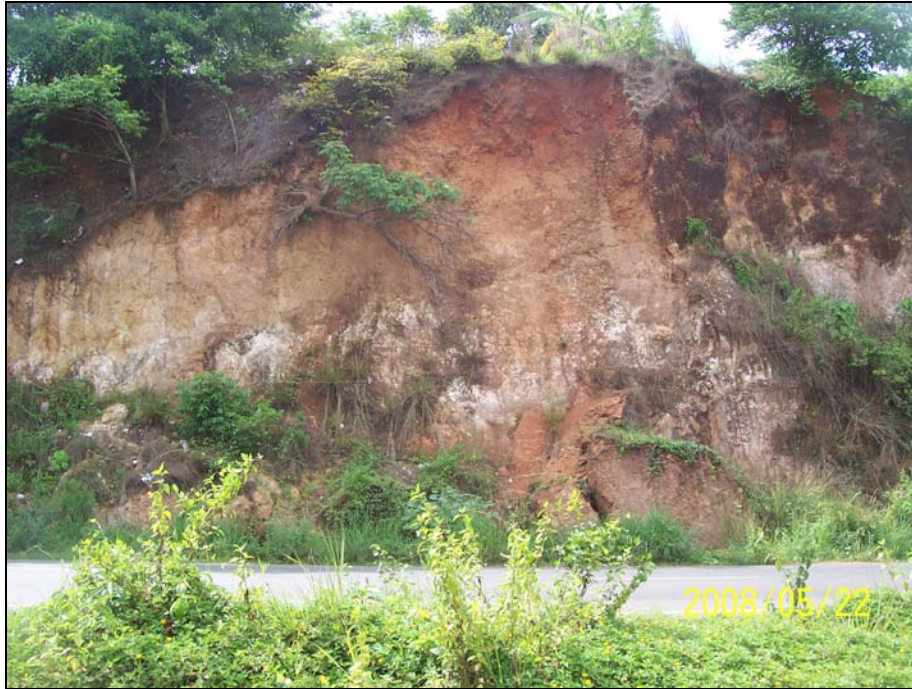
Photo 119: The plan view of the debris slump with unstable crown
