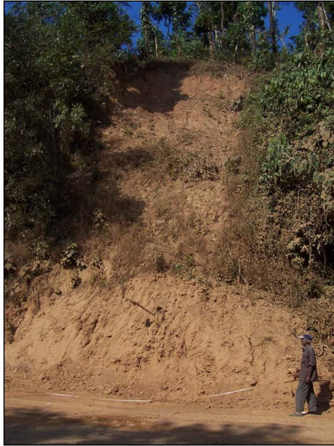
Photo 32: The plan view of the debris slide with unstable crown
