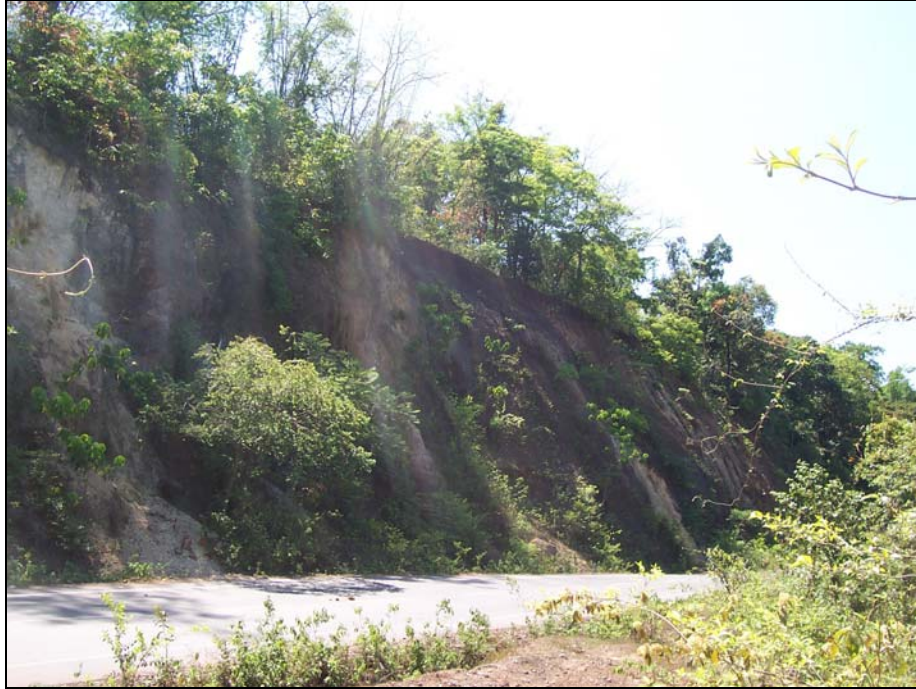
Photo 92: The side view of the debris slide
