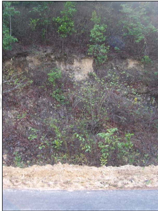
Photo 63: The plan view of the reactivated rock slide along day lighted plane.
