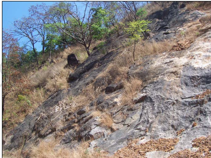
Photo 75: The side view of the rock slide
