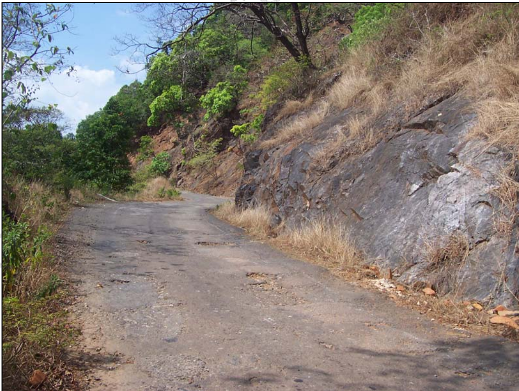
Photo 85: The side view of the rock slide.
