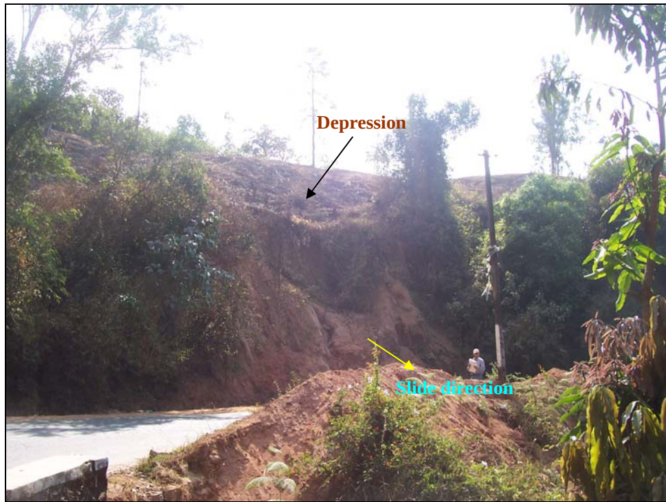
Photo 11: The view of the slide with the depression on the slope.
