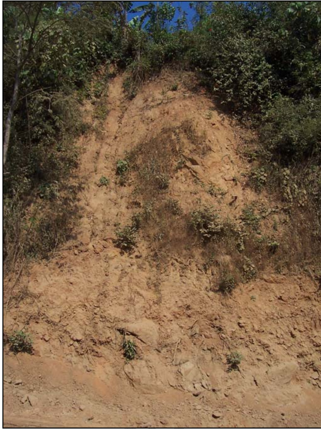
Photo 30: The plan view of the debris slump
