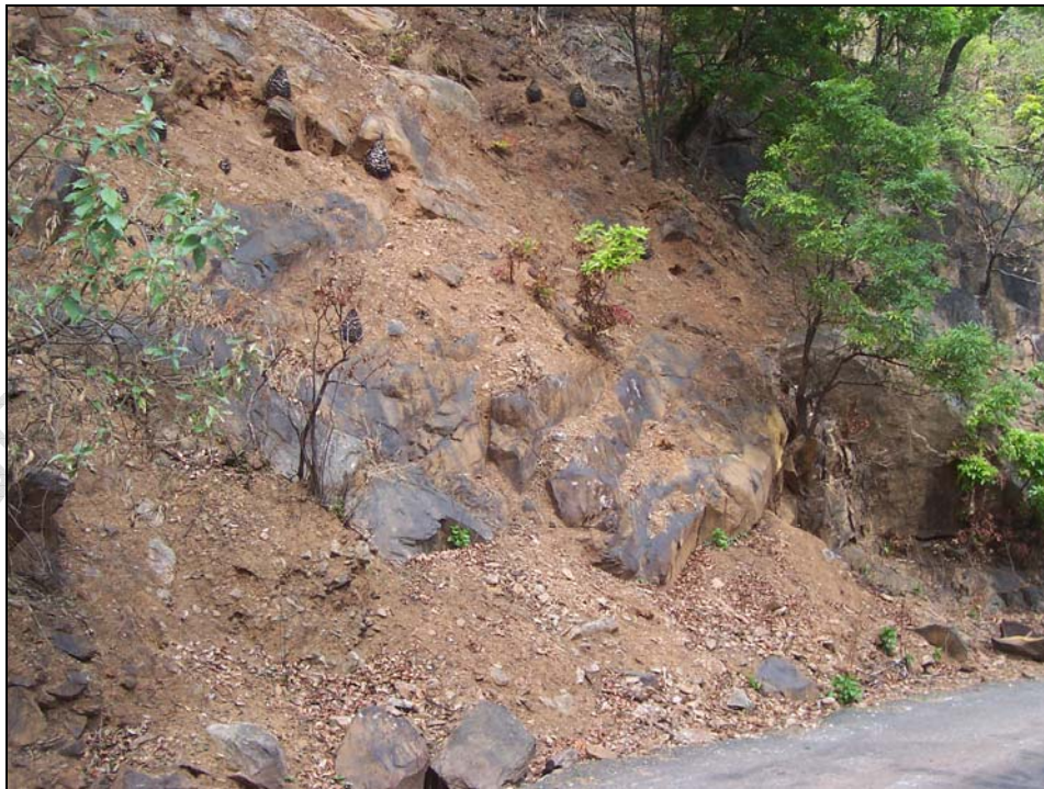
Photo 83: The view of the rock slide.
