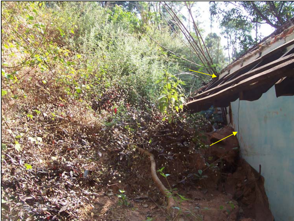
Photo 8: The debris accumulation and damage to the back wall and roof of the house.
