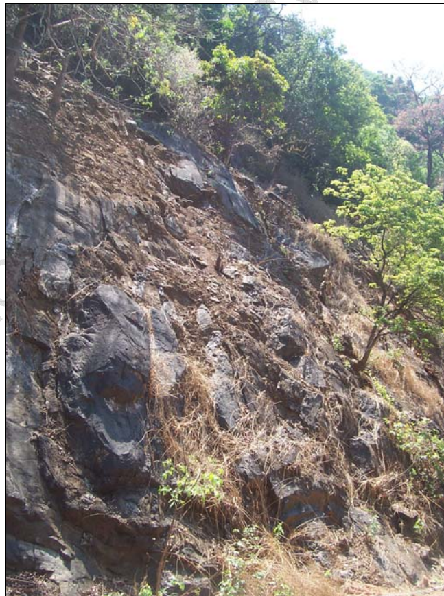
Photo 79: The view of the slide plane of rock slide.
