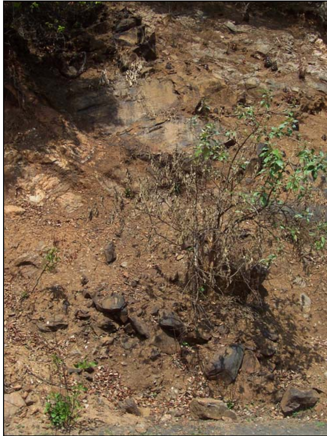
Photo 82: The view of the debris slide with unstable crown.
