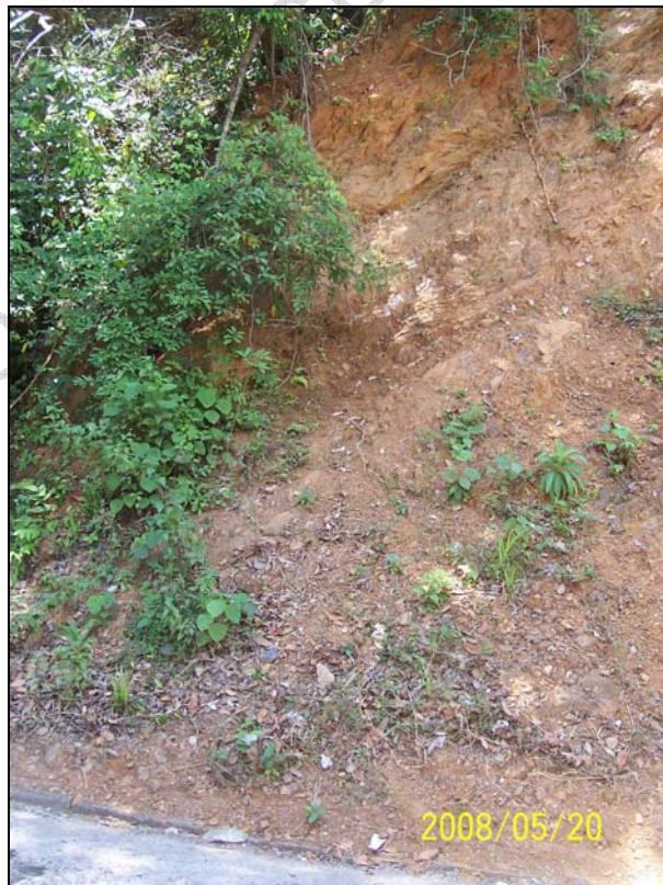
Photo 118: The side view of the debris slump
