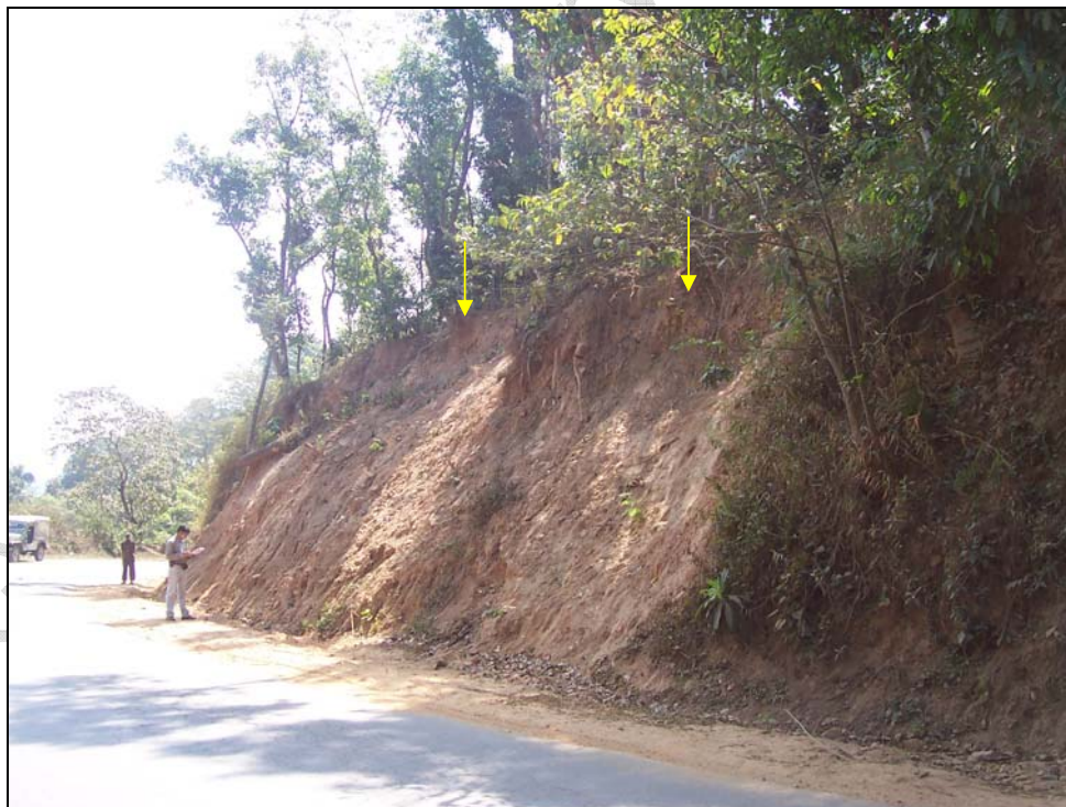
Photo 20: Two sources of the shallow slide on the cut slope along SH88
