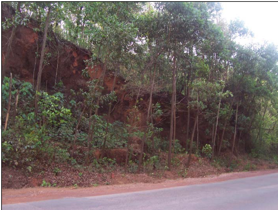
Photo 109: The side view of the debris slide showing steep slope angle.
