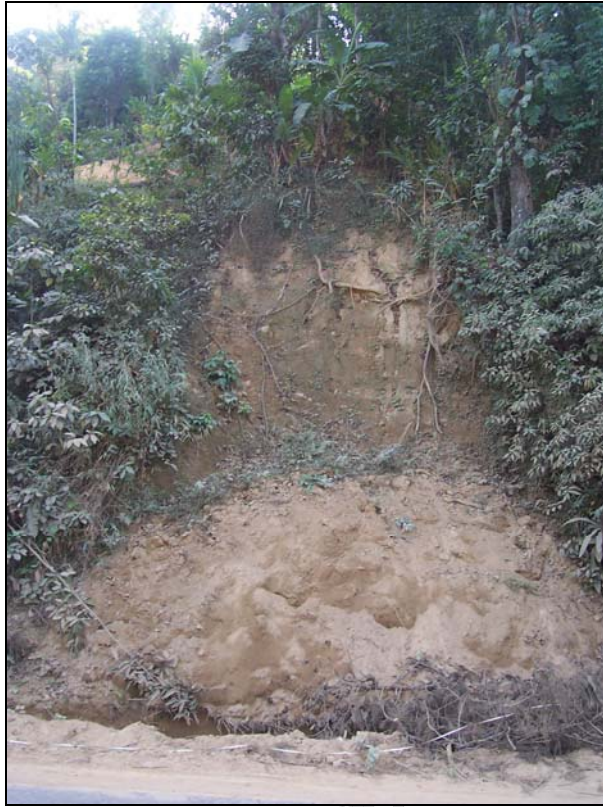
Photo 38: The plan view of the debris slide with unstable crown
