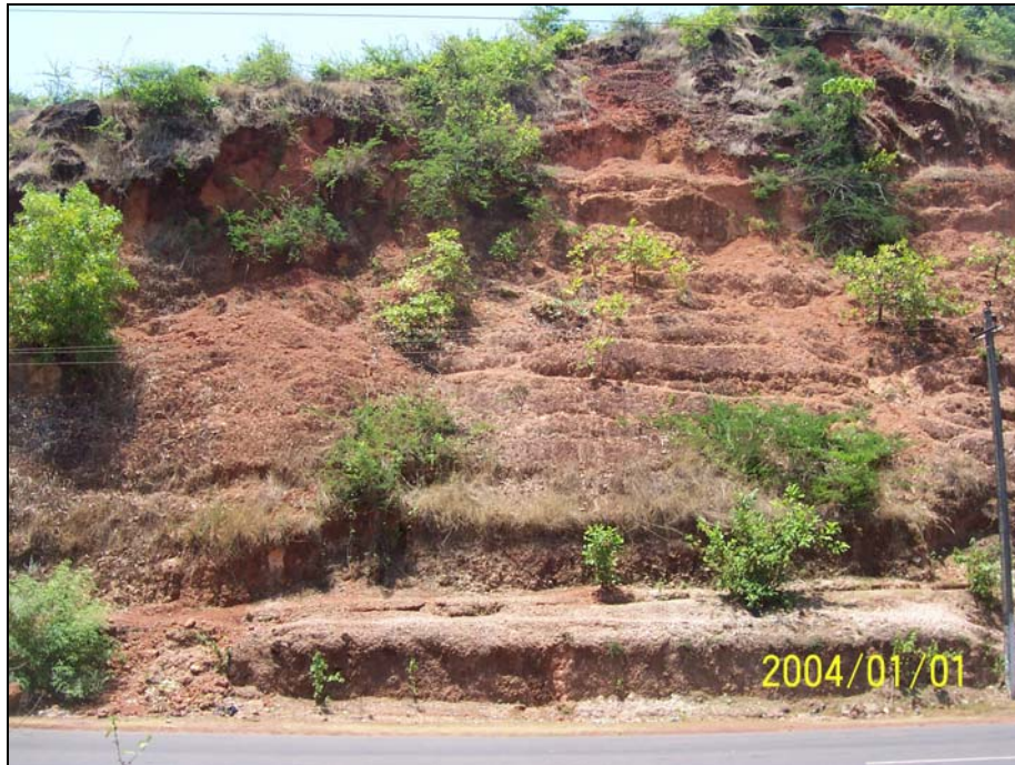
Photo 125: The plan view of the reactivated, debris slide with unstable crown
