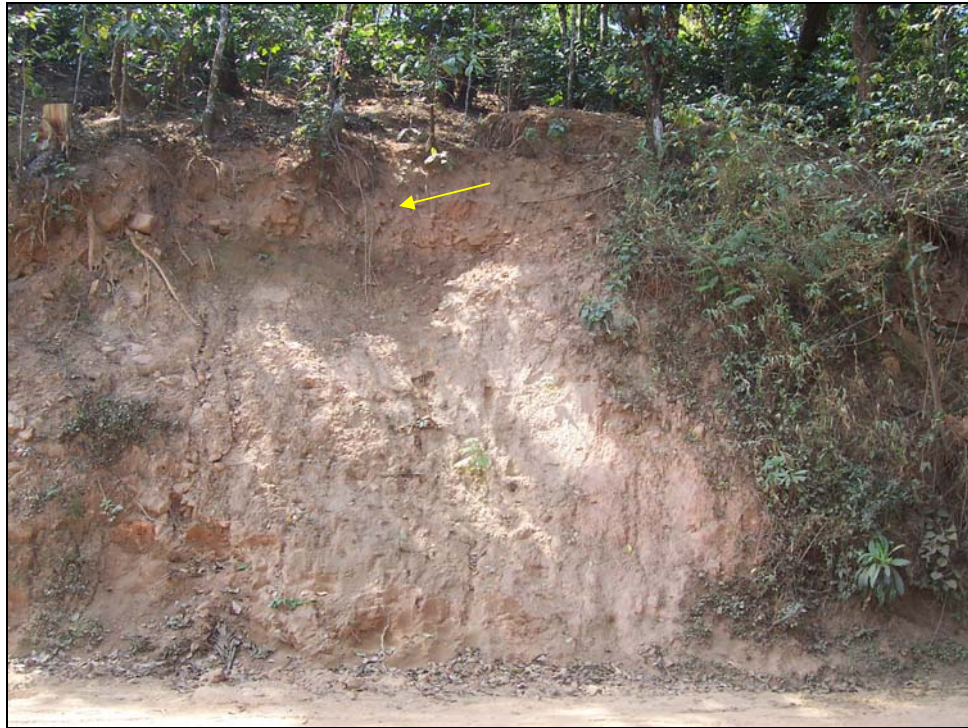
Photo 19: View of the landslide along the cut slope of SH88
